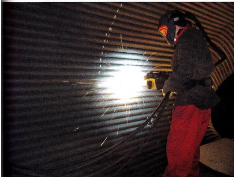
Fig. 1. Area coated by Arc Spray Technique (rear and roof membrane walls and suspension tubes).
